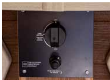
Ignition and Flame Controller
